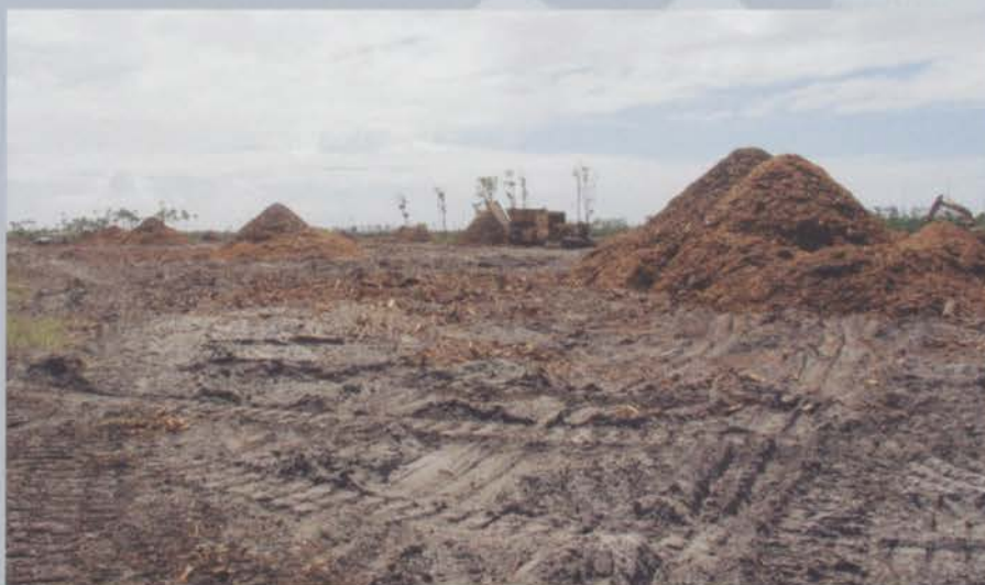
Preparing the site for the new Pacific Harbour course at Bribie Island has begun
