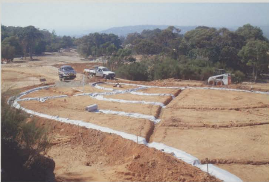
Construction of a USGA spec green at Elanora Golf Club in NSW
