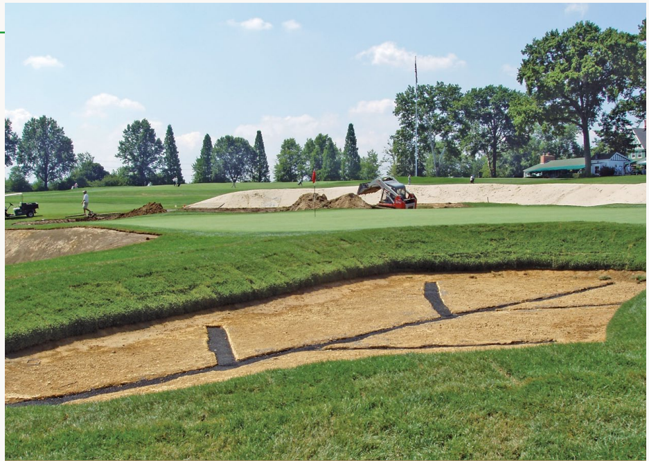
A large portion of the restoration work is targeting the course's 190-plus bunkers
