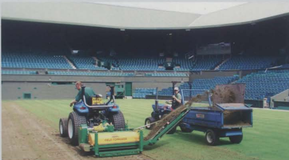
Renovation of all courts begins immediately after The Championships. Here the Koro field topmaker is used on Centre Court
