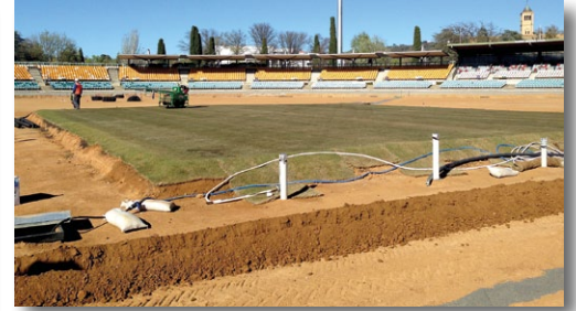
The new seven deck wicket table was turfed with maxi rolls of washed Legend couchgrass
