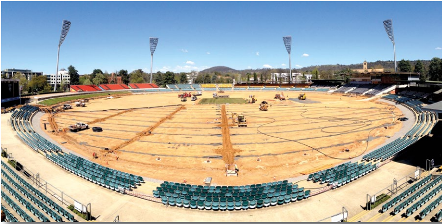
The herringbone drainage system was installed with 100mm ag pipe at 6m centres
