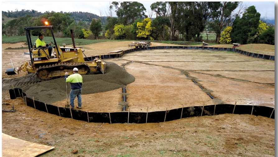
Installation of the gravel layer. A poly membrane barrier has been installed around the perimeter of each green
