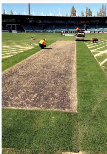
The drop-in pitch was installed in two halves utilising a 100 tonne crane and two flat deck semi-trailers. Transformer turf was then installed around the edge of the pitch
