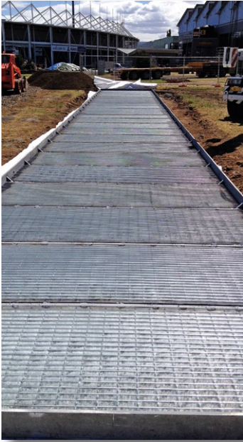
Fabrication of the pitch frame started in the first week of April 2013. Mangalore clay, sourced just north of Hobart, was used as the wicket soil for the Aurora drop-in
