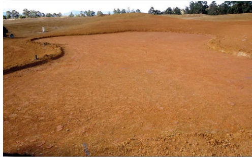
Being on an old clay quarry, there was no shortage of site material to construct the compacted clay bases
