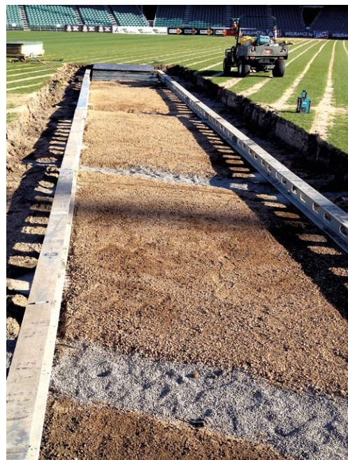
Construction of the base in the centre of the main arena started in late September 2013. The base consisted of 20 concrete piers, eight 200mm steel 'I' beams and sand and gravel to match the existing Aurora outfield profile
