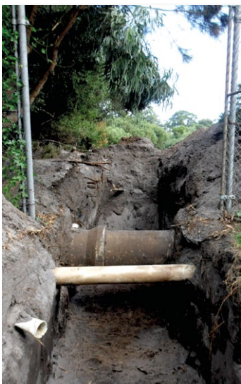
One of the main challenges for the installers was a 400mm diameter 'barrel drain' which runs diagonally through the course
