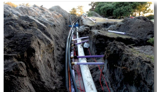
With four separate mainlines to install, an excavator was required to create trenches wide enough to accommodate some 45km of pipe
