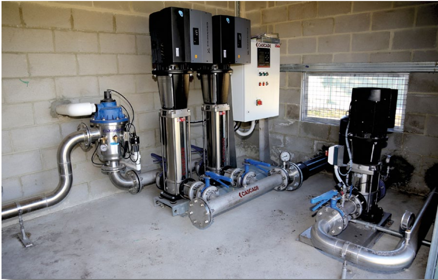
The new pump shed (installed as part of the sulphur-treated system) comprises two Grundfos Hydro pumps as well as circulation pump (right) to circulate water between the tanks and the sulphur burner
