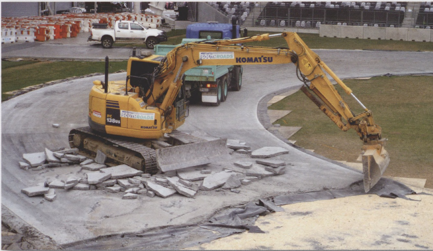
The morning after the event, two diggers with bucket attachments came in and started breaking up the concrete track
