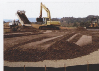
Both the sand and gravel should be tested together in the lab for compatibility to ensure the gravel will support the sand layer above
