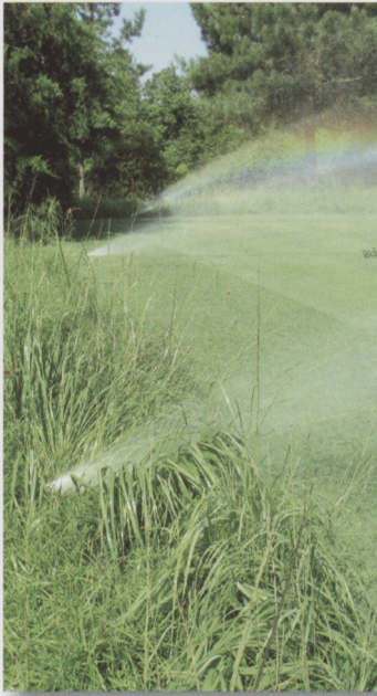
Turf can grow over sprinklers and disrupt irrigation coverage, especially in rough and naturalised areas. Check and trim turf around sprinklers every month
