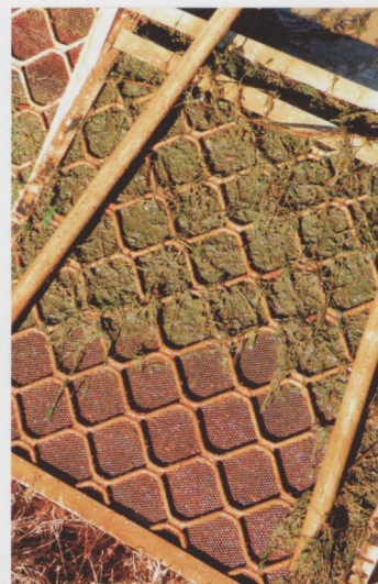
Algal blooms, which blocked screens and restricted flow to the wetland pumps, were among a number of teething problems which had to be overcome early on in the system's operation
