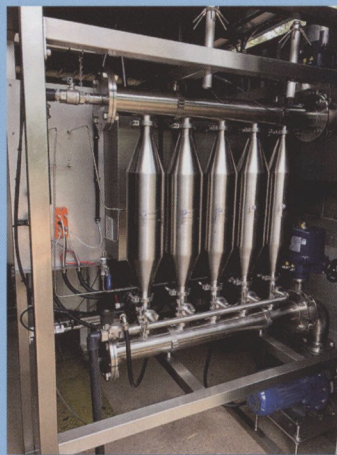
The new Nano Bubble Technologies unit installed at Avondale Golf Club
