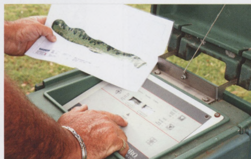
Checking the satellite controllers and central computer for backup programmes and accurate run times should be done at least once every month
