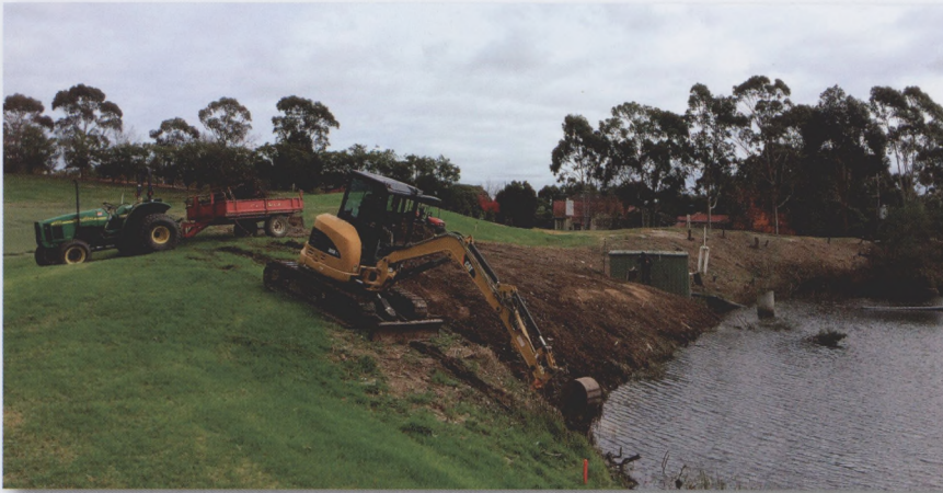
An excavator was used to remove 200mm of weed seed infested topsoil and to create a smooth batter for jute matting to go down
