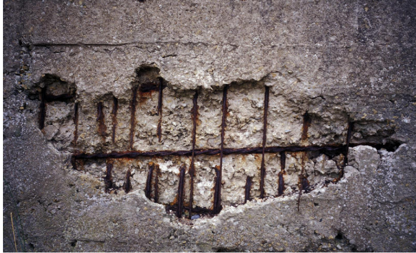
Figure 1.1: Steel Corrosion in Concrete. For interpretation of the references to color in this and all other figures, the reader is referred to the electronic version of this thesis.
