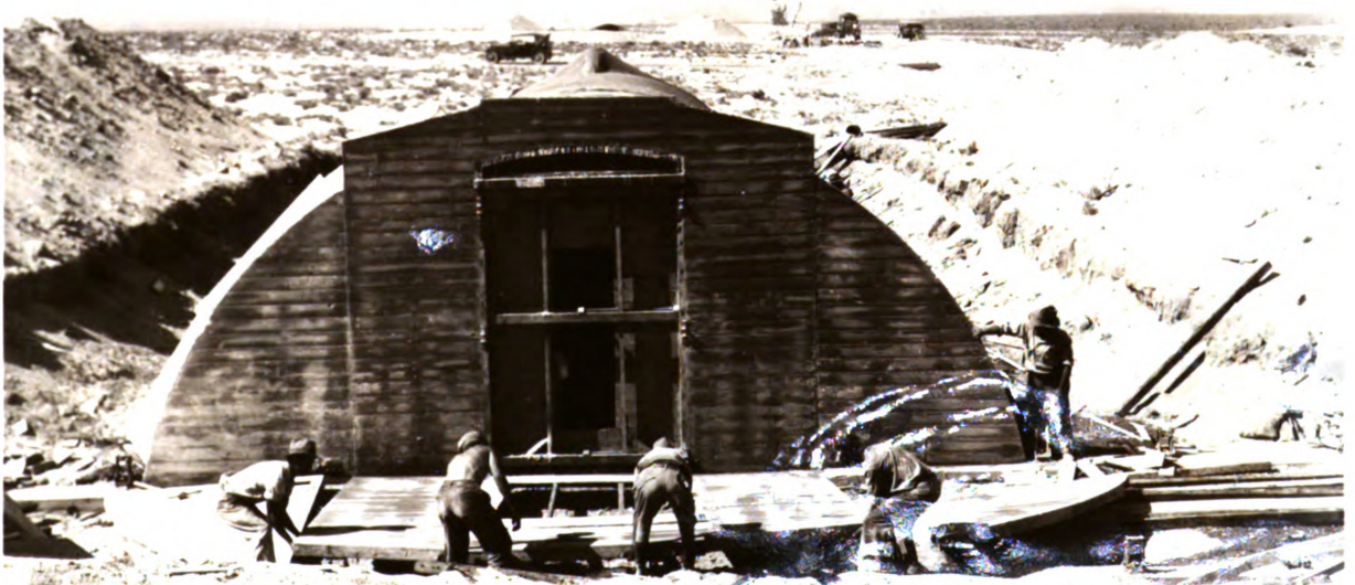
Example of excessive roughness due to warped boards in forms
