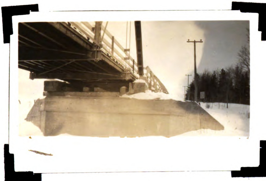
This view shows lateral movement which has taken place in North Abutment.
