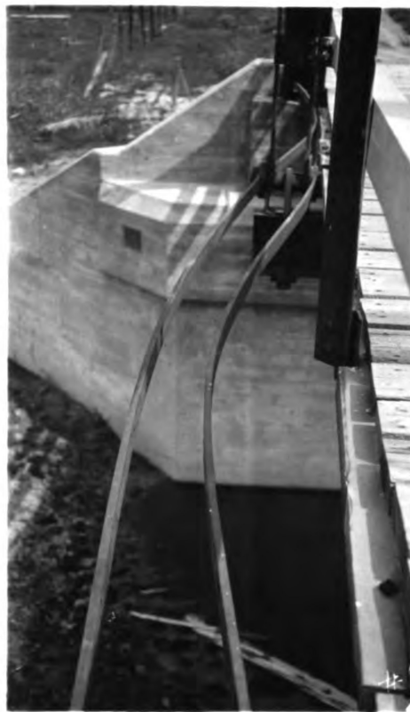
This view shows buckled lower chord, and has been repeated many times.
