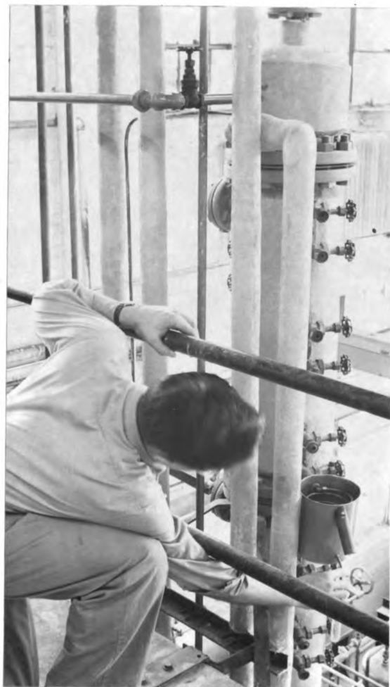
Figure 7. Sampling apparatus, showing the valves, unions and cooling coil.
