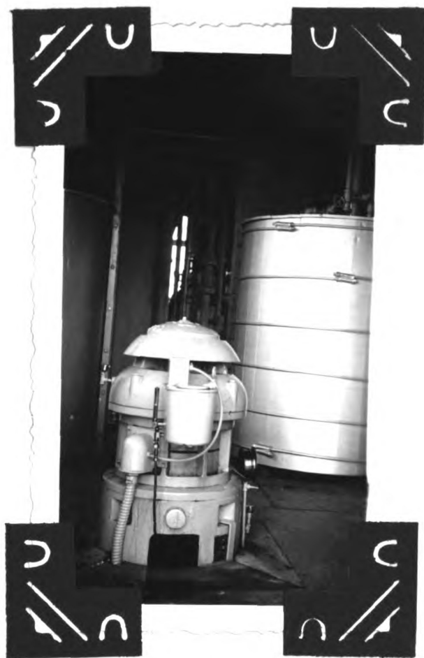
Well pump motor Well # 1
