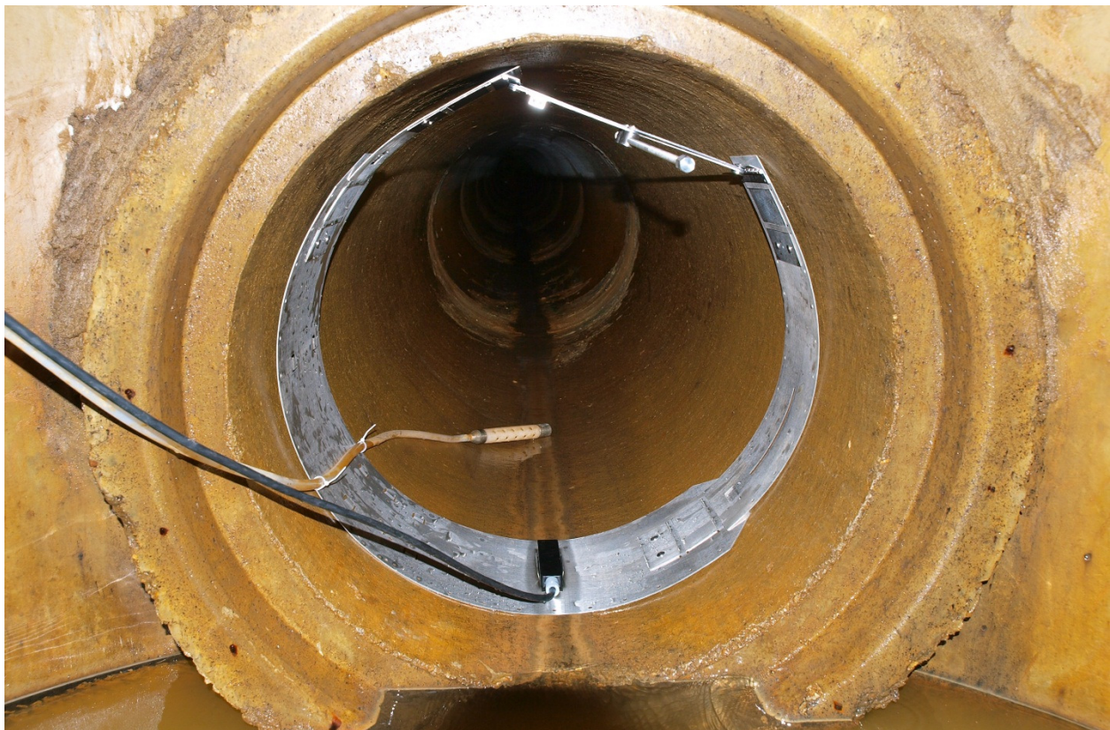
Figure 10 Area 750 Velocity Flow Sensor at the Bioretention Basin
