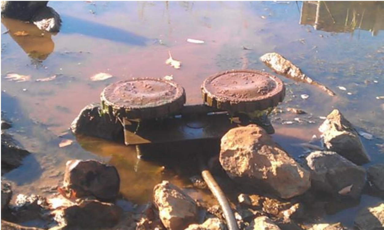
Figure 14 Vertex, Pond-Lyfe 1 Aerator
