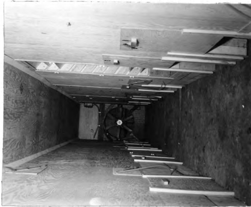
Fig. 6. View of Main Duct Showing Air Control Gates and Slatted Wall Section.
