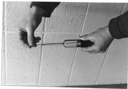
Figure 4.5. Air indicator and a metal wire used to scour out the mortar.
