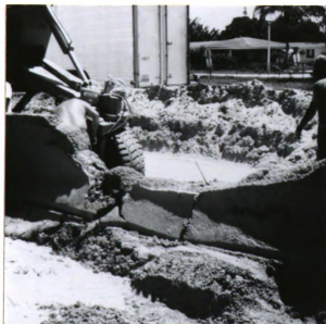
Figure 1.2. A slump failure of the fresh concrete structure.
