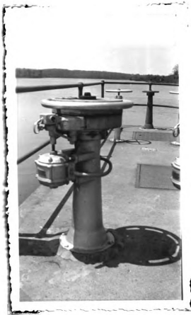
Left: View of downstream valve control wheel at the Geddes Plant. The small motor turns the wheel. A button-switch in the power house controls the motor. The upstream valve wheels are shown in the background. They are for emergency use only as pressure is usually maintained by water entering the chamber between the idler and the upstream leaf.
