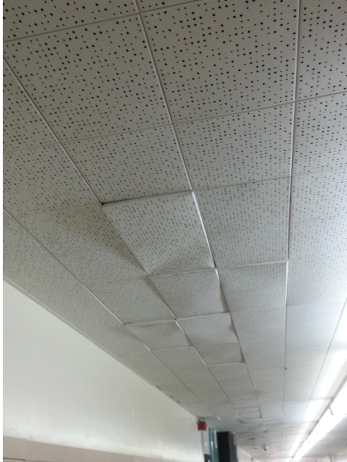
Figure 5.1. Photograph: Uneven ceiling tiles at Murphy.
