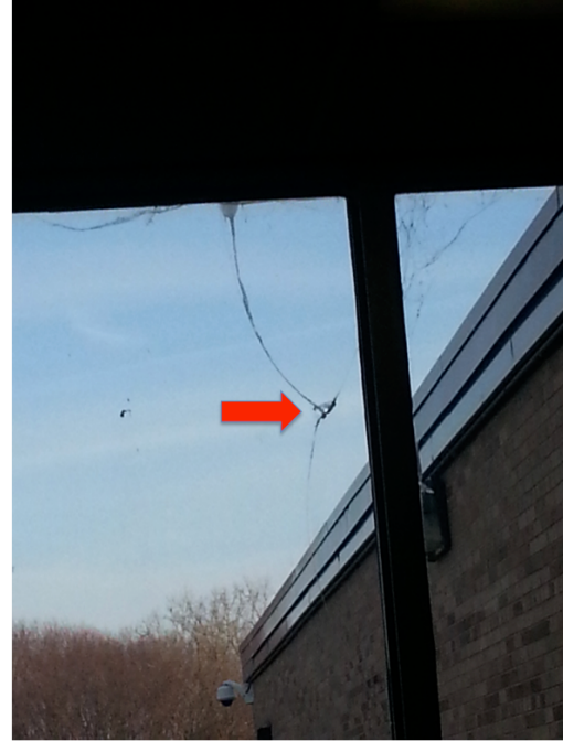
Figure 5.2. Photograph: Hole in window at Murphy.
