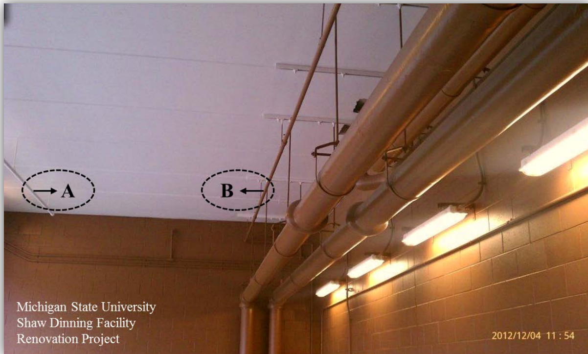
Figure 4.18 – Incompatible Pipe Color Coat
