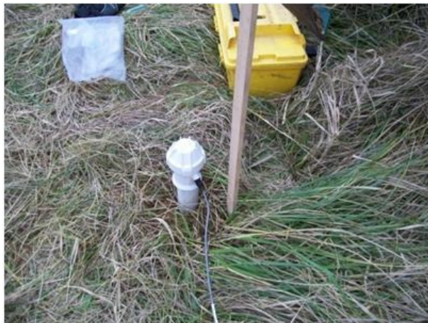
Figure 3-16 Installed enviroscan sensor.
