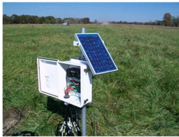
Figure 3-13 A station showing solar panel, datalogger, cables and battery.
