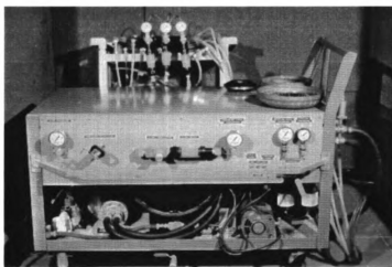
Figure 3. Transmission Oil Supply System
