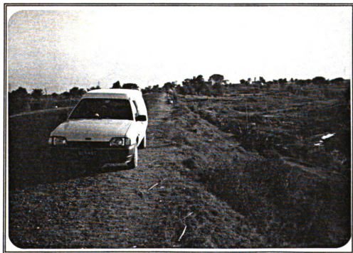
Deficient Shoulder Width: Hazardousness Evaluated by MOH [SWIDTH].
