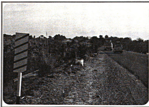
Deficient Guardrail: Hazardousness Evaluated by MOH [GDRAIL].
