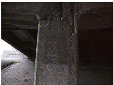
Figs. 5.1 Column condition before surface repairs
