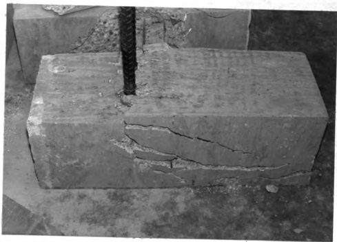
(c) Spalling of Concrete Cover.
