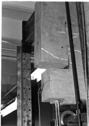
Figure 3.24: Split Cracking Resulting From Dowel Bars Acting Against Cover.
