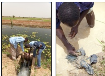
Figure 12: Poor maintenance of ON irrigation canals
