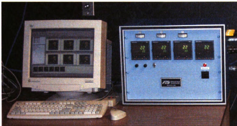
Figure 13. Computer and ATS Controller.
