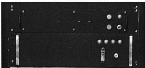
Figure 8.12. Data conditioning hardware, motion control and power supplies.
