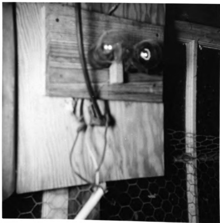
Fig. 54. The two other fan motors used in the house required two bulbs in the time of operation instruments, one for the low speed and one for the high speed. The thermocouple is attached to the bulb which is in parallel with the high speed winding of the motor.
