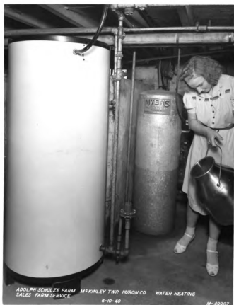
Fig. 16. An electric water heater in the basement provides a constant supply of hot water in the house. Automatic time switches are generally provided in electric water heaters. (Courtesy: Detroit Edison Company)
