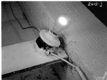
FIG. 67. A poorly installed lamp is a hazard. Faulty installation should be guarded against. (Courtesy: Michigan State College)
