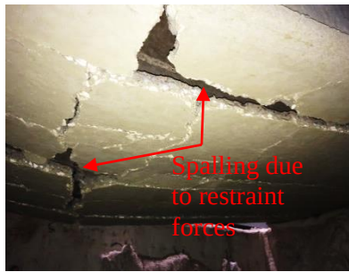
b. Slab 5, spalling
