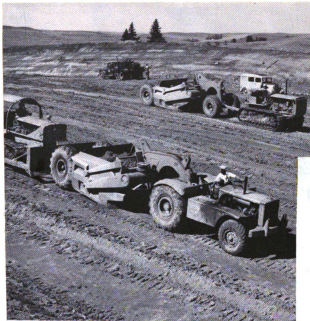
Part of R. A. Heintz's "Caterpillar" Zoned Equipment fleet, building highway near Moscow, Idaho. In the background a D8 pulls a "Caterpillar" No. 80 Scraper on a medium-length haul. The scraper in the foreground is being push-loaded by a D8. In a moment the "Caterpillar" Diesel DW10 Tractor will roll off with it to a distant fill.
