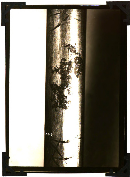
FIGURE SHOWING CORROSION OF STEEL.
