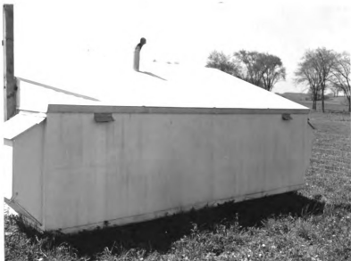
Figure 17. A rear view of one of the houses showing the air intakes and the exhaust duct through the roof.
