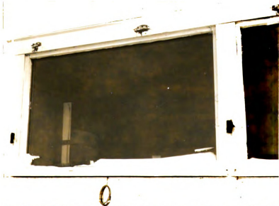
Figure 33. The double-pane windows never had any frost on them but moisture did condense on the inside surface.
