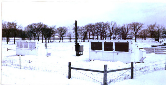
Figure 31. A typical view on cold mornings showing how the single-pane windows frosted over while the double-pane windows did not.
