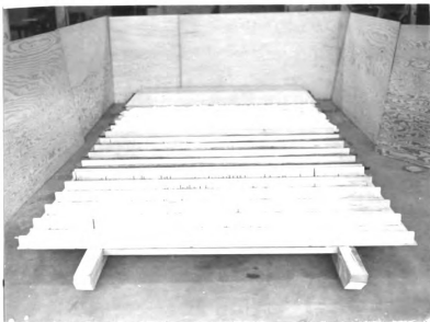
Figure 11. The four stages of the construction of the roof and floor panels.
