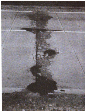
Figure 3-1. Typical Transverse Joint Failure
