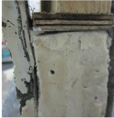
Figure 8.6 Damage mechanism during shear failure of the ferrocement skin-aerated concrete core interface with shear connector
