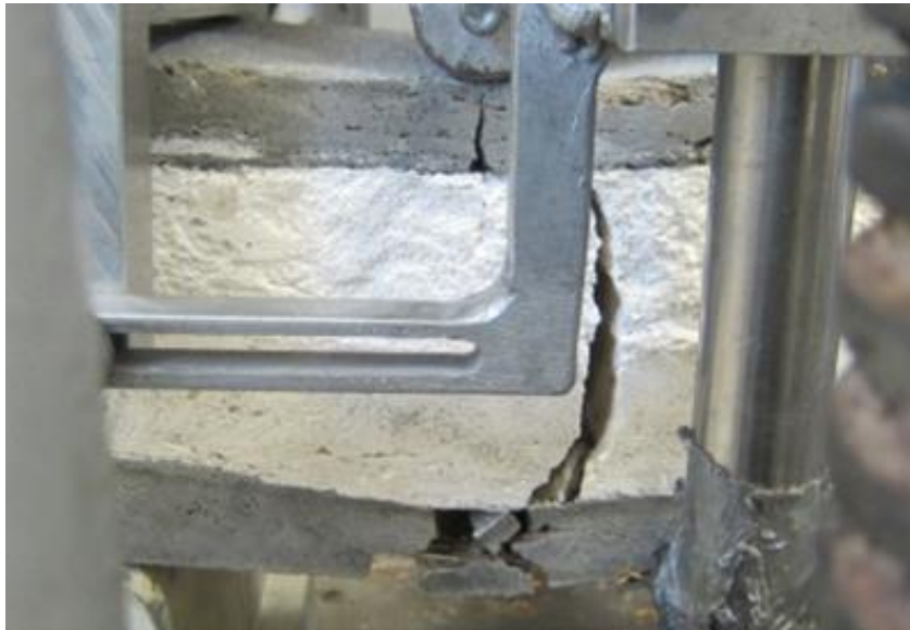
(b) Failure by rupture of the lower skin followed by full-depth cracking of sandwich composite
