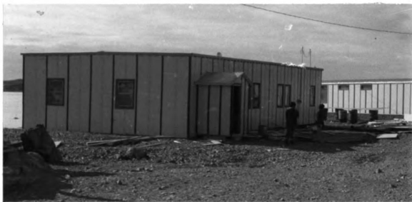
Figure 21. Construction of the New Co-op Retail Store with Office Building in Background.
