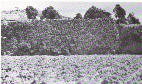
Plate 13a Particularly high terrace wall in Bashut. This wall collapsed and was reconstructed at least twice. Due to levelling of the flat below the wall further destruction may occur.
