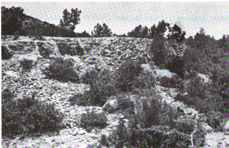
Plate 12a Abandoned dry-field terrace in the southern part of Bashut, near Al-Habil village east of the new road. Note the collapse of any part of the wall will lead to the collapse of the whole wall and the wash of terrace soil.
