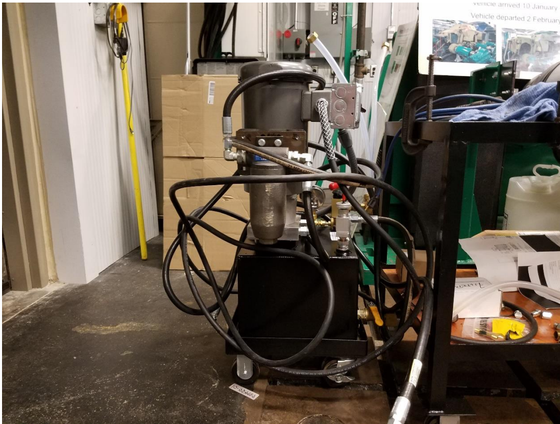
Figure 1: Hydraulic pump and hoses
