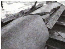
Figure 3.21. Brittle Failure of Unreinforced Pipe
