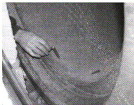
3.20. Crack Width Measurement
