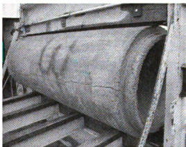
Figure 3.19. Global View of Second Horizontal Crack
