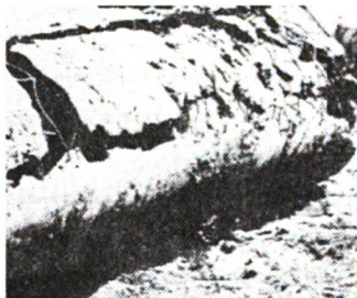
Figure 1.1. An Example of Damage to Reinforced Concrete Caused by Microbial-Induced Corrosion.
