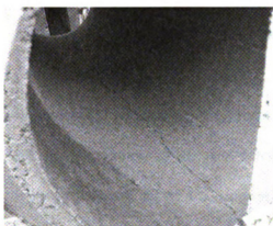
Figure 3.17. First Vertical Crack Inside of the Pipe
