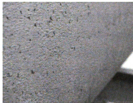
Figure 3.18. Second Horizontal Crack Outside of the Pipe
