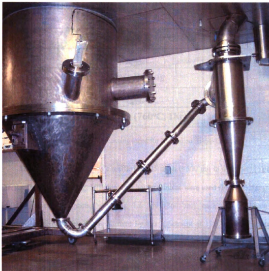
Figure 3.4. Ti atomization tower and cyclone at Crucible Research Corporation used to make Ti-64-1B powder via pre-alloyed approach. The height of the room is about 5 m. [Yolton (2007)]
