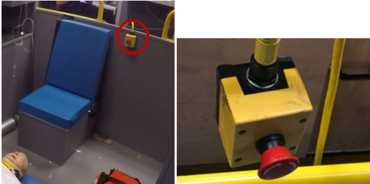
Figure 59. Mechanical E-stop nearby captain's seat
