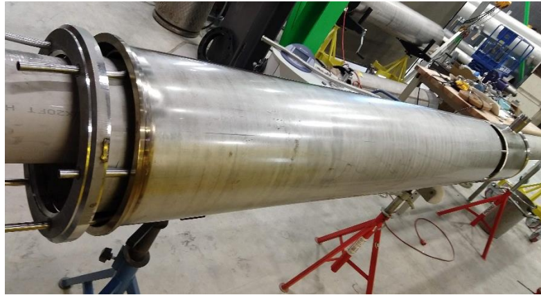
Figure 4.5: Heat exchanger with shell installed
