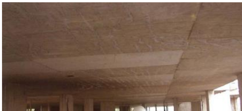
(a) Thermal crazing (cracking)
