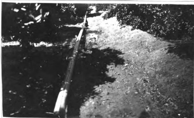
Portable galvanized pipe conveying water to basins.
