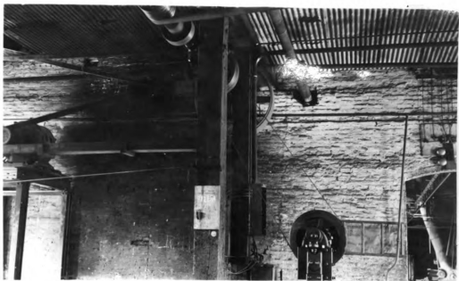
Fig. 6. Machine shop motor showing belting to line shaft. Switch box on column by punch press is shown in Fig. 8.
