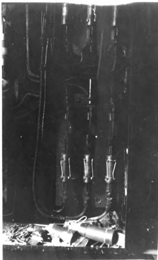
Fig. 5. Reinforced fuses on branch circuits in service cabinet and remains of some blown fuses. Due to unequal resistance of the several current paths it is almost impossible to estimate the capacity of such a makeshift and therefore they are over fused, thus loosing all benefit of fuse protection.
