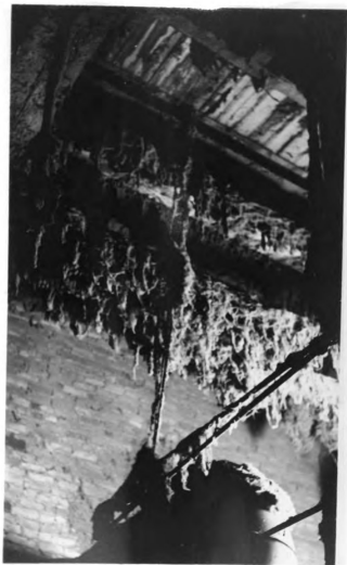
Fig. 19. Slag Festoons on wires near cupola. Illustrating why wires should be in conduit.
