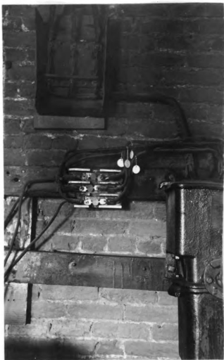
Fig. 18. Tumbler motor switch, fuses and starter. The switch is upside down. The cutout arrangement is a very serious hazard for the wires are sprung into the old clips and if one wire was pulled loose and short-circuited with either of the others the only fuse protection would be at the service switch and on the high tension side of the transformers. The renewable fuse links are mechanically very weak. The slightest pull breaks them causing loss of productive time.
