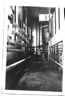
View of Piping System.
