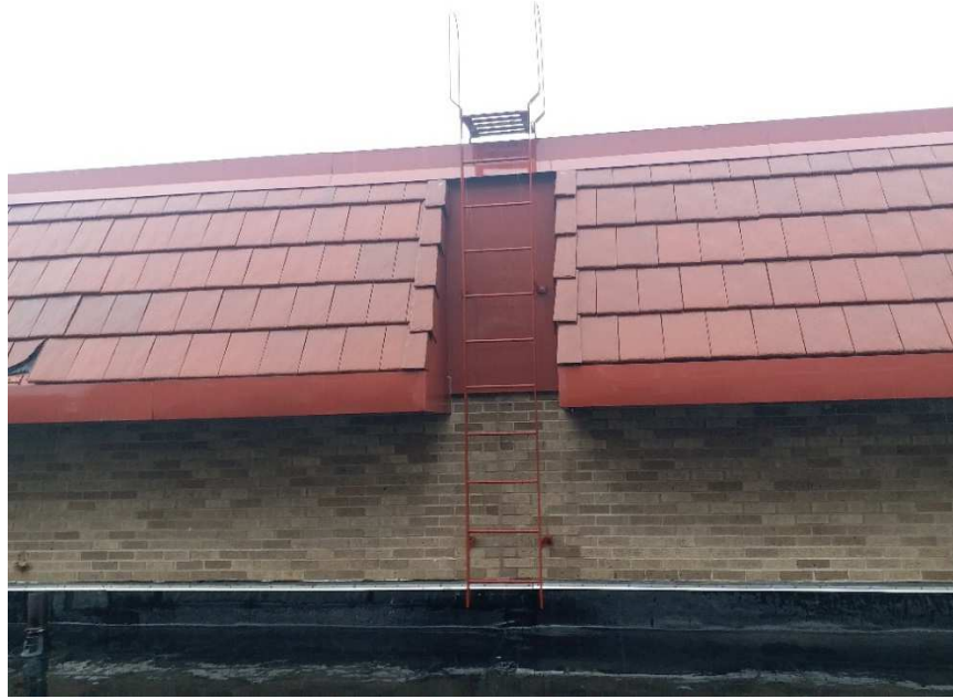
Figure 5: A latter giving access from level two to level three roofing. (Copyright © 2019 Wing Chi Vincy Tam all right reserved used by permission).
