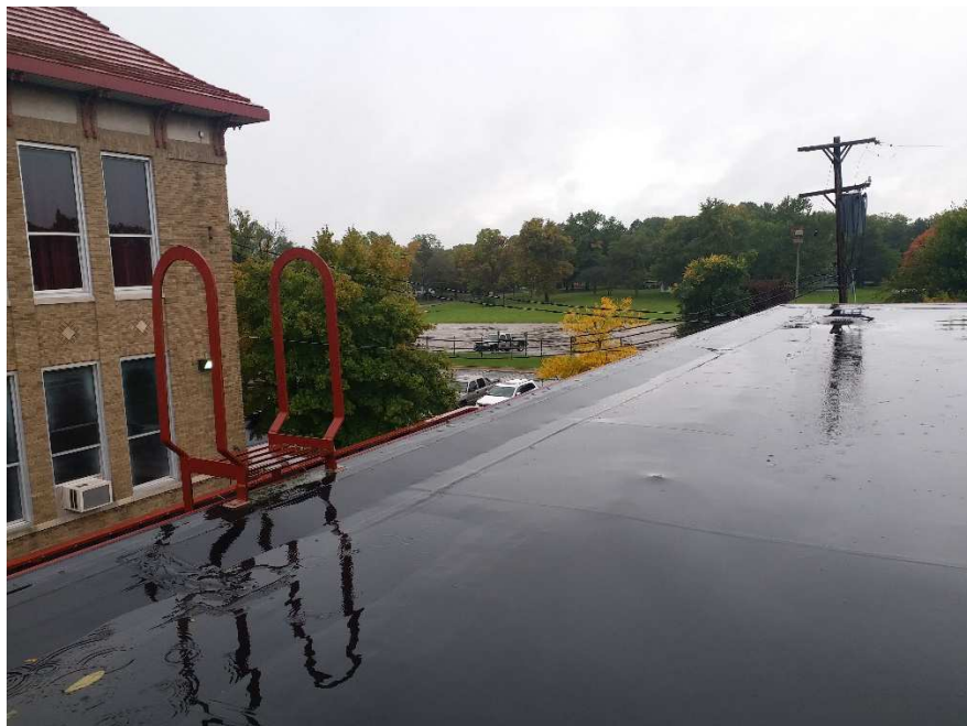
Figure 6: No railing on level three rooftop. (Copyright © 2019 Wing Chi Vincy Tam all right reserved used by permission).
