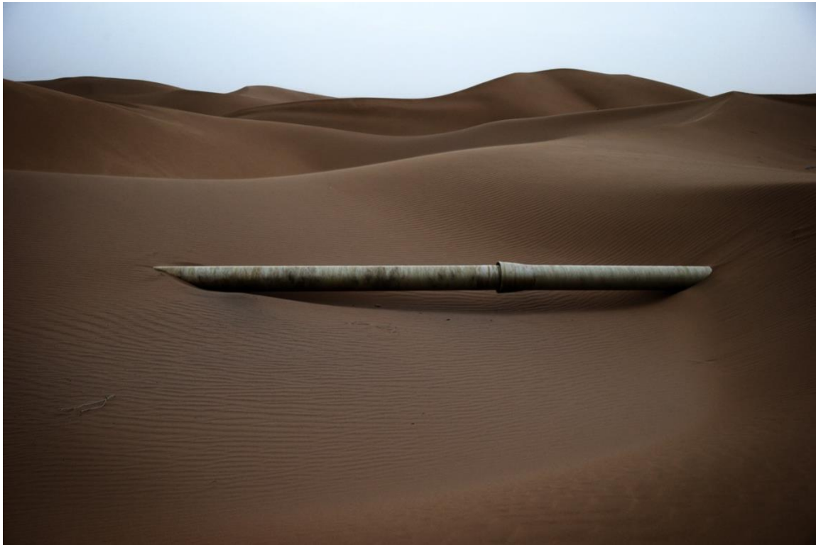
Figure 11. From the industrial park to the evaporation ponds, a white glass fiber reinforced plastic sand pipe stretches two miles through the desert and continuously poured untreated wastewater into the evaporation ponds. Provided by Chen Jie.
