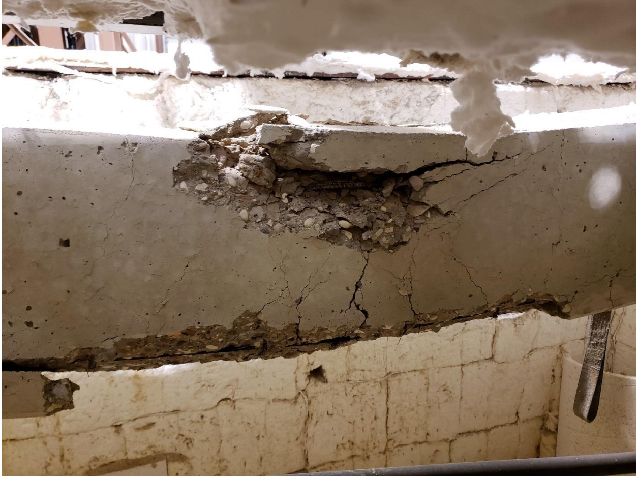
Figure C.4 Cracking and crushing of concrete in beam N1R after failure
