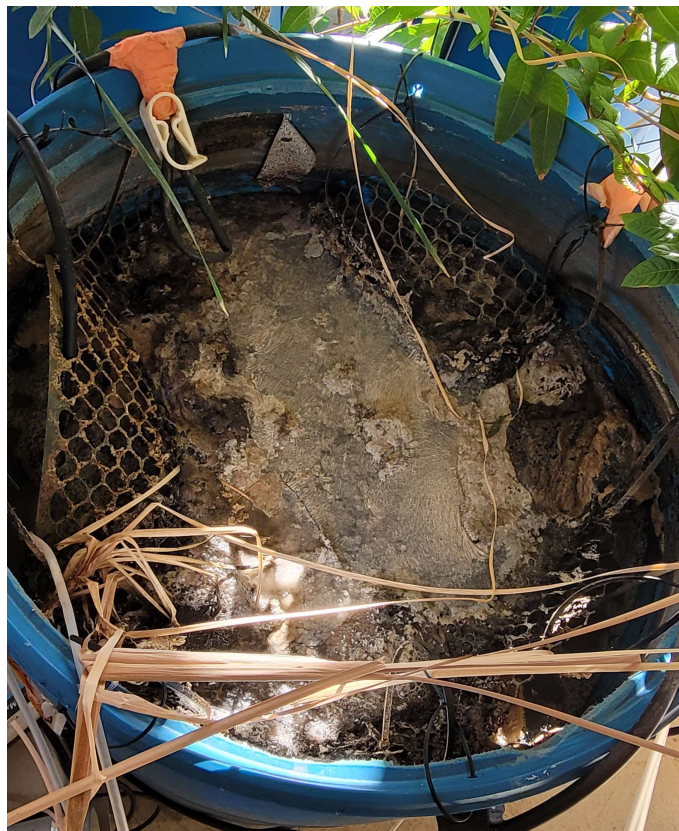
Figure 8: Train 2 Reactor 1 with brewery wastewater film on top of water surface.
